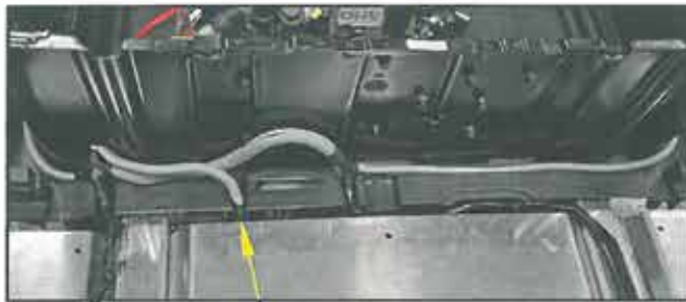
Main wires FNR wires go below floor
